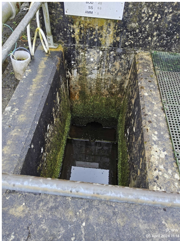
Photograph 3: DCWW no-flow evidence 05 April 2024
