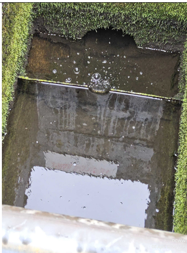
Photograph 4: DCWW no-flow evidence 05 April 2024
