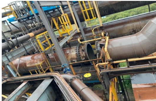
Photo: Blast Furnace Gas supply to Boiler 3 decommissioned
