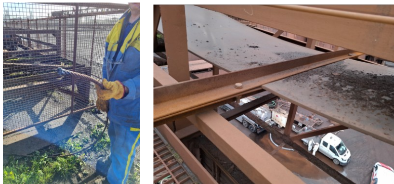
Photo: dead weights cable cut, conveyor belt secured
