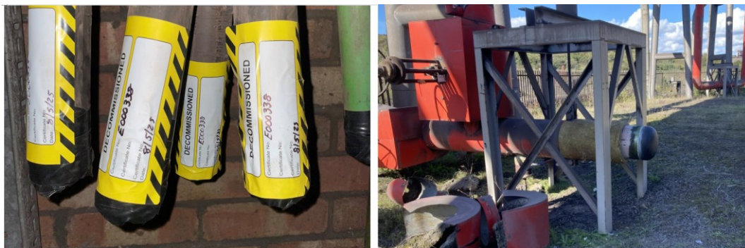
Photo: no 6 TA electrical cables cut and capped and 11 bar steam superheater capped
