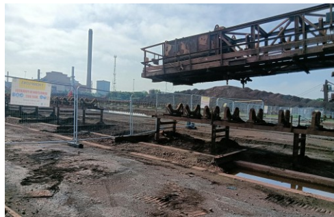
Photo : section of conveyor structure removed in stockyard area for CDM perimeter fencing.
