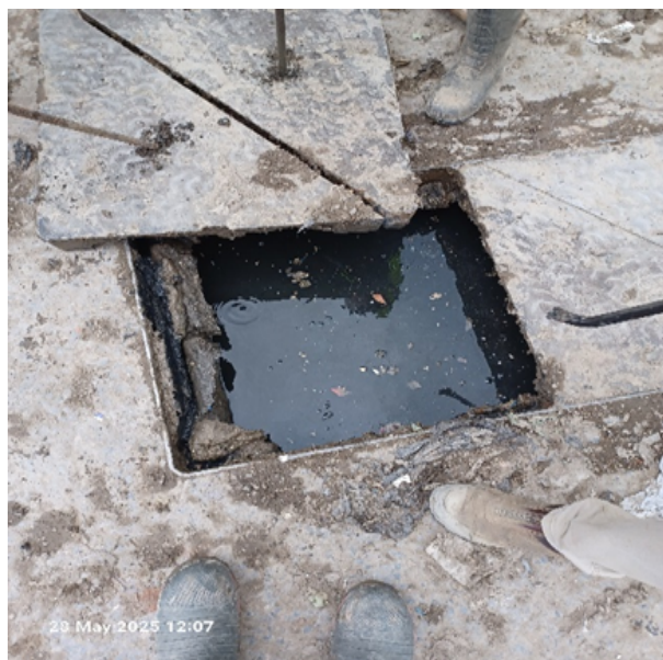
WTS drain sump
