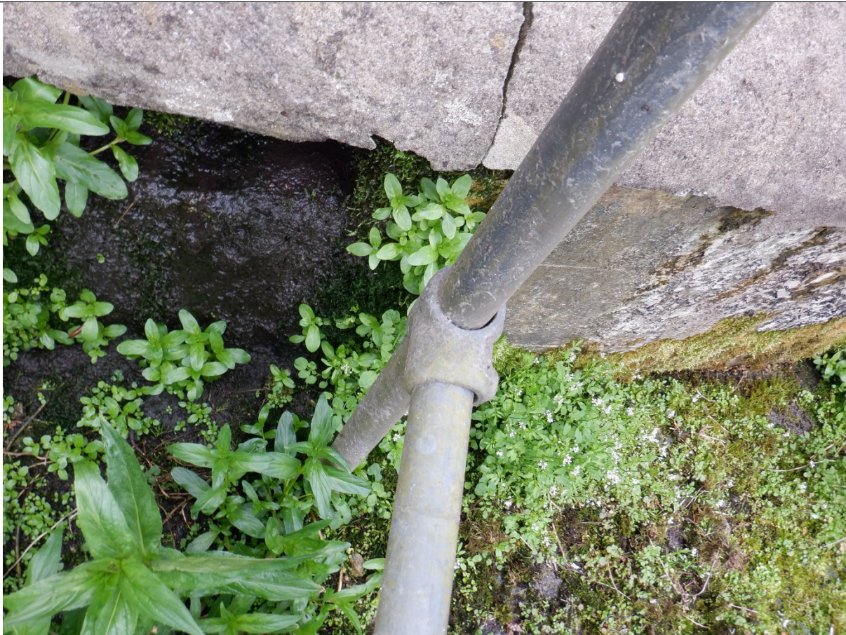
Figure 2: Leak from final settlement tank wall.
