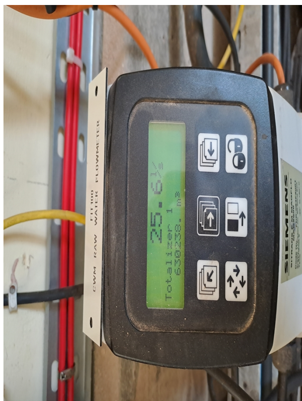
Figure 3 – The meter digital display at the time of the visit.
