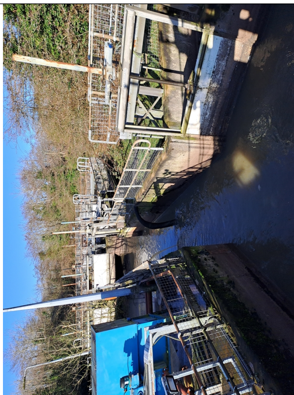
Figure 9 – Large black pipe as observed during the visit.
