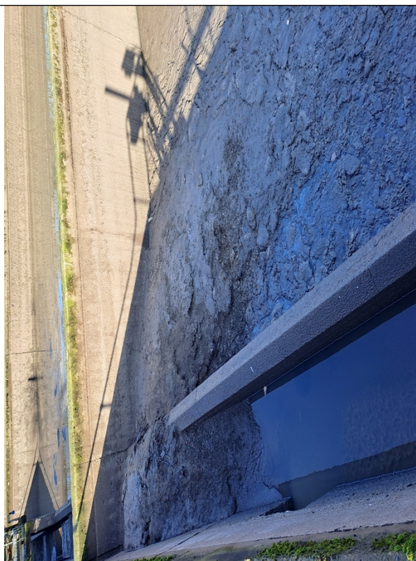
Figure 18 – Significant sludge buildup at the inlet of Storm Tank 3.
