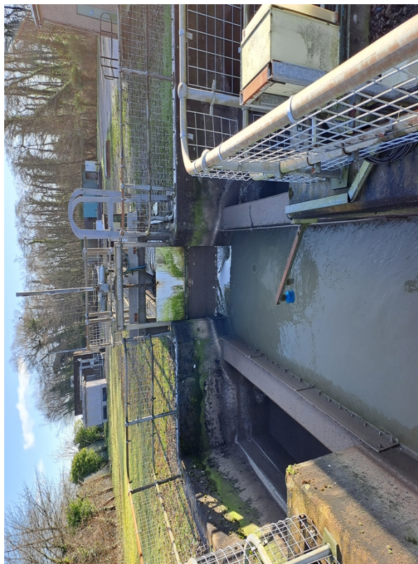
Figure 6 – Storm overflow weir with sensor visibly in place.
