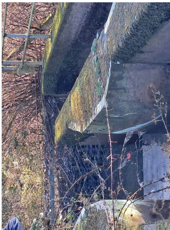
Figure 22 – Final screen prior to storm outfall blocked by debris as observed during the visit.
