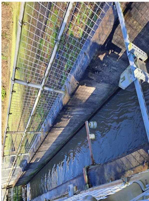
Figure 12 – Level sensors observed to be in place on the flume
