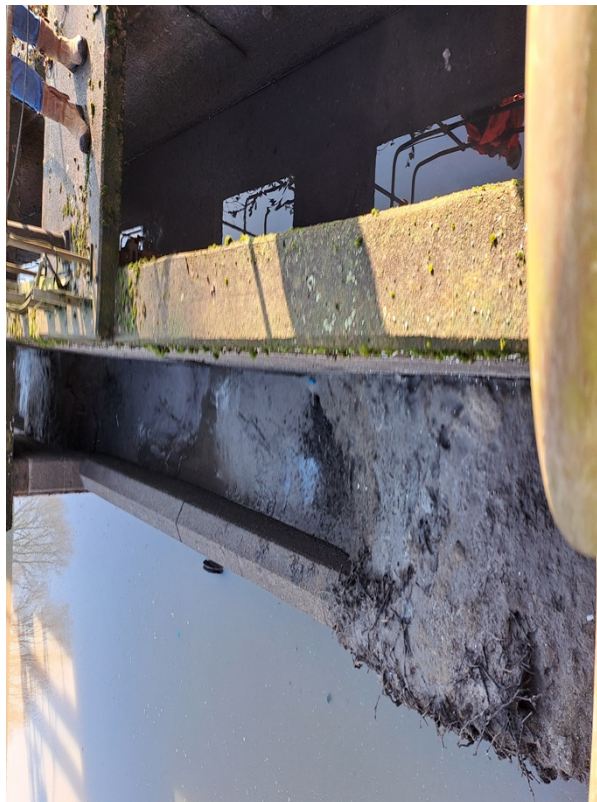
Figure 14 – Sludge buildup at the inlet of Storm Tank 1.
