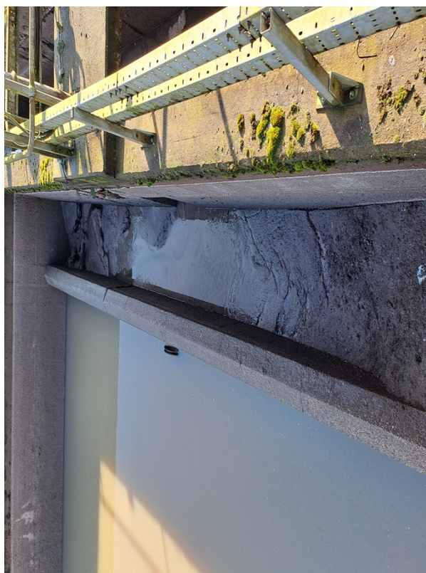
Figure 16 – Sludge buildup at the inlet of Storm Tank 2.
