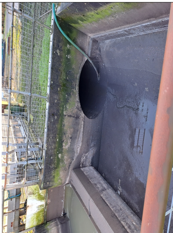
Figure 7 – Storm overflow outlet to the storm tanks.
