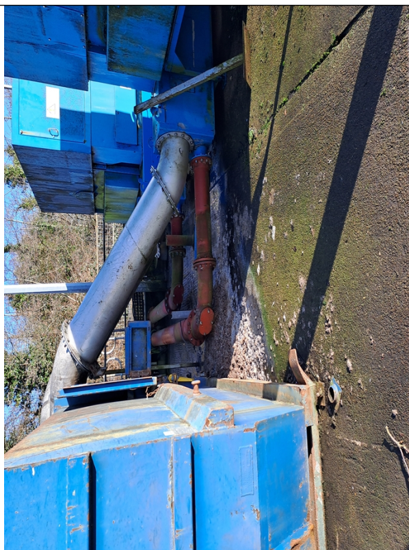
Figure 4 – The on-site waste skips with the escaped wastes collecting beneath them as observed during the visit.
