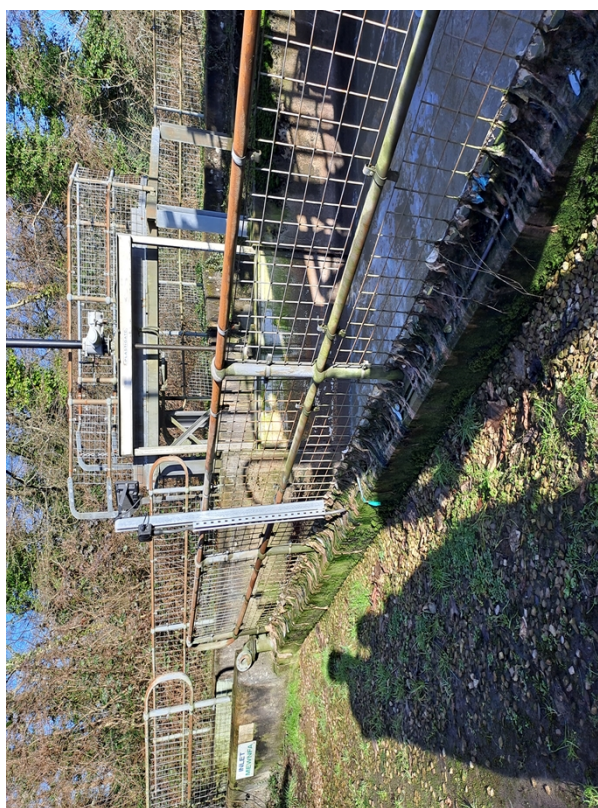
Figure 1 – Ragging and debris buildup on the safety railings showing evidence of a spill/overflow at the site.
