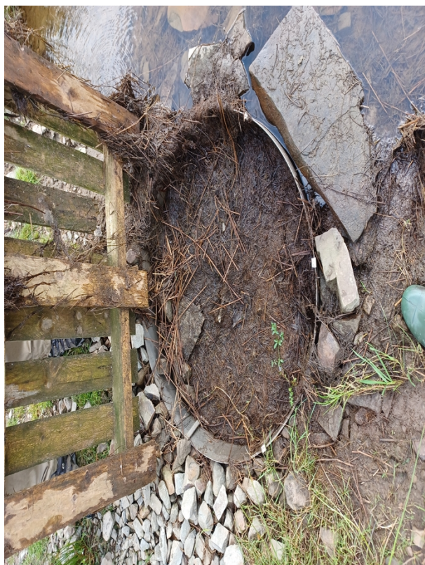
Image 1: Concrete ring structure clogged with dead vegetation
