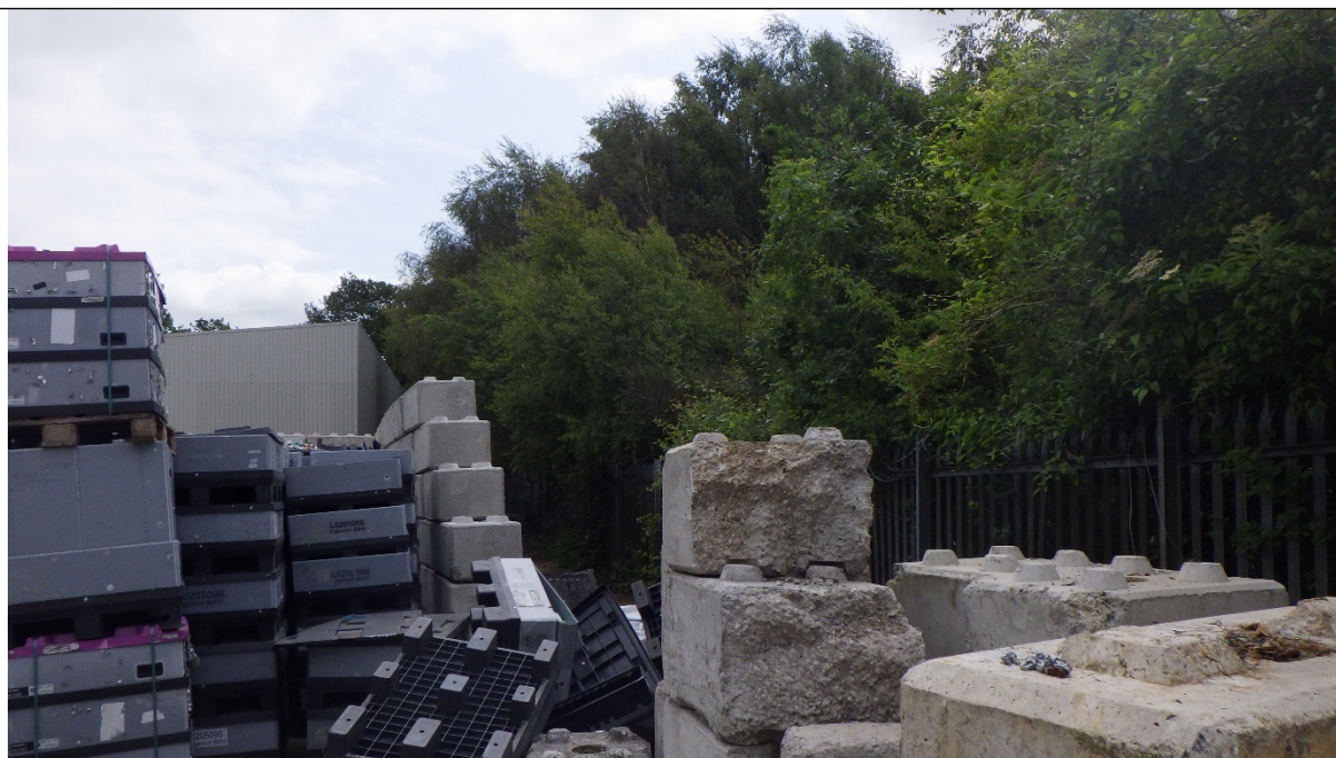
Photograph of acoustic wall not completed at rear of site.
