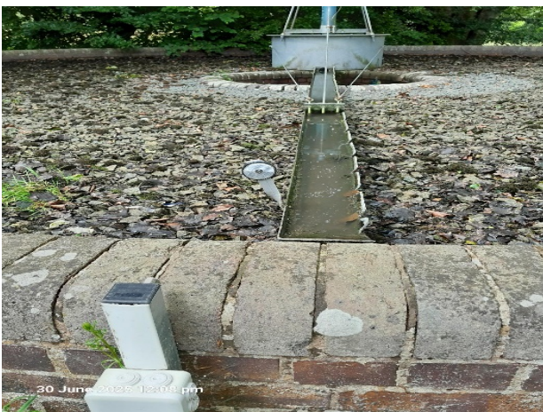
Image 4 – filter bed cracks
