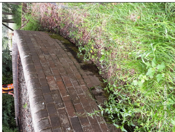
Image 5 – Final effluent chamber had growth
