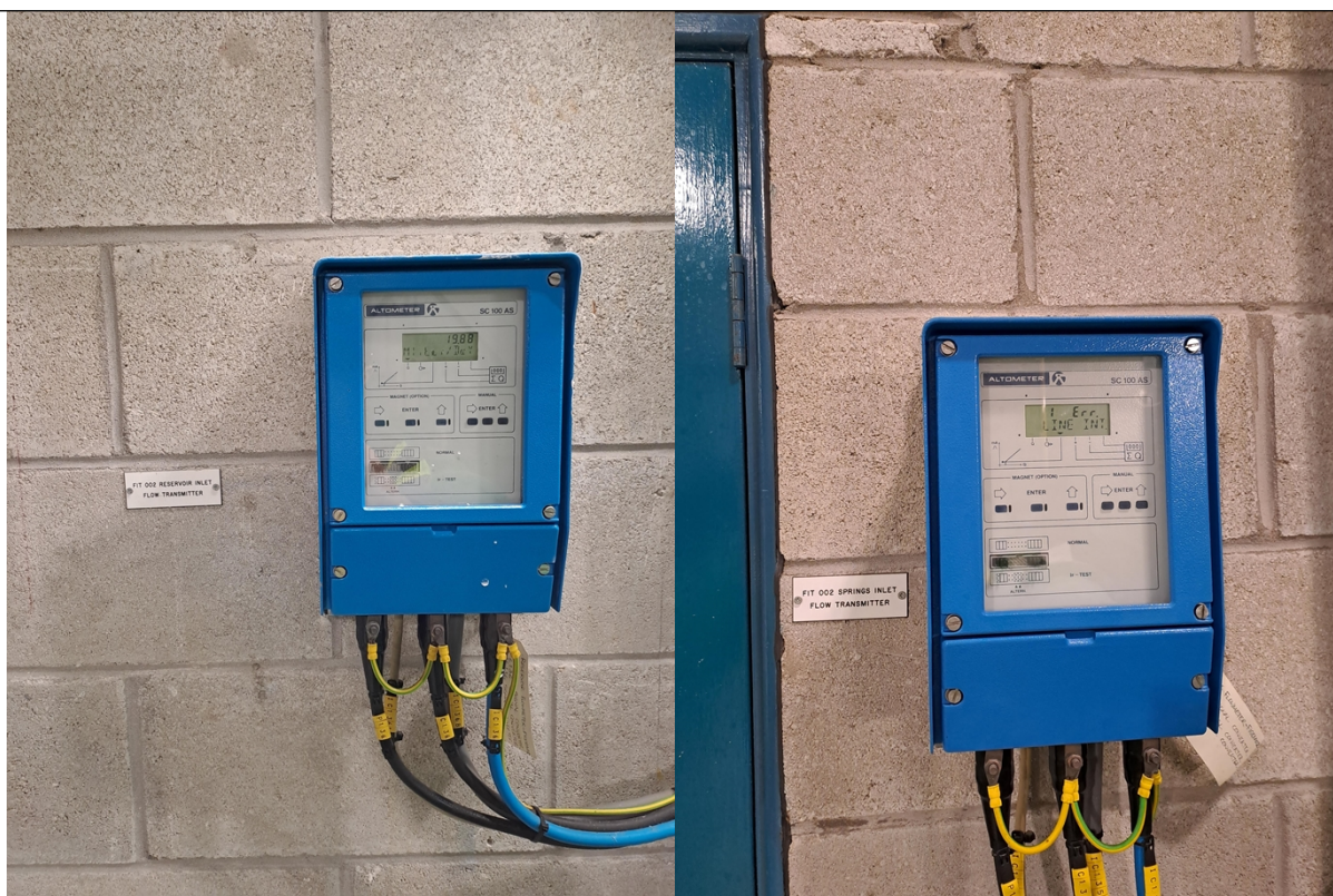
Figure 2 – Meter readouts as observed during the visit.
