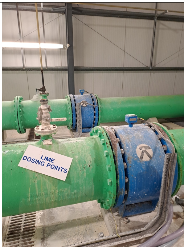
Figure 1 – Flow meter heads observed within the control building. The far meter head is for the spring, the close meter head is for the works.
