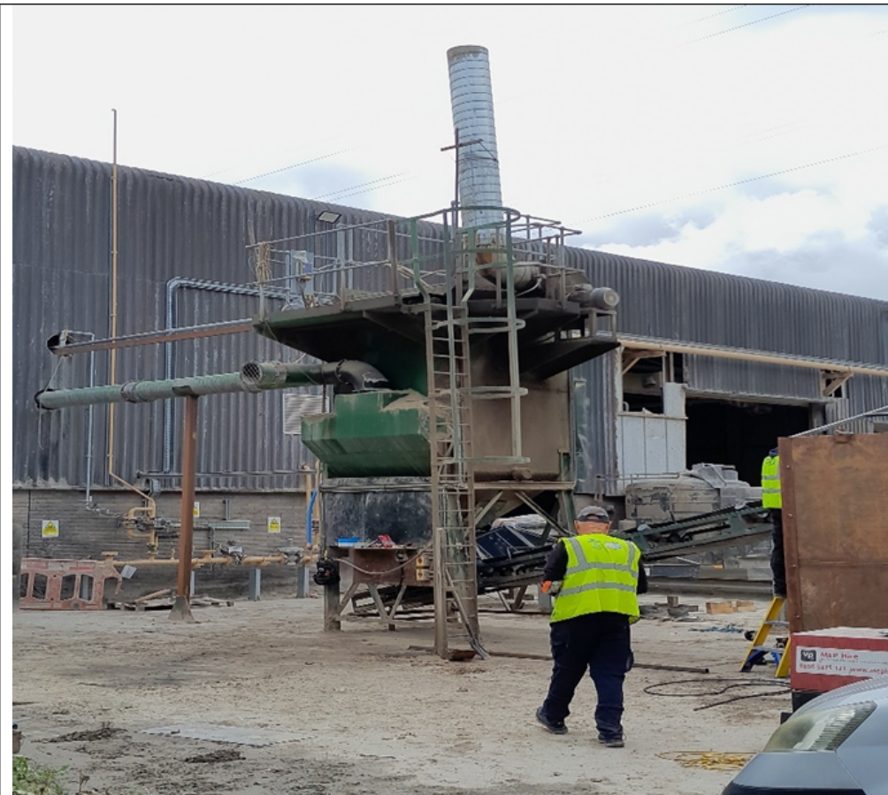
Photo1 – showing engineers servicing the dryer outside.
