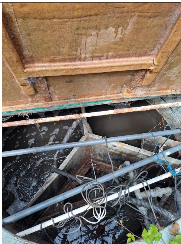
Figure 4 – The treatment system as observed during the visit.
