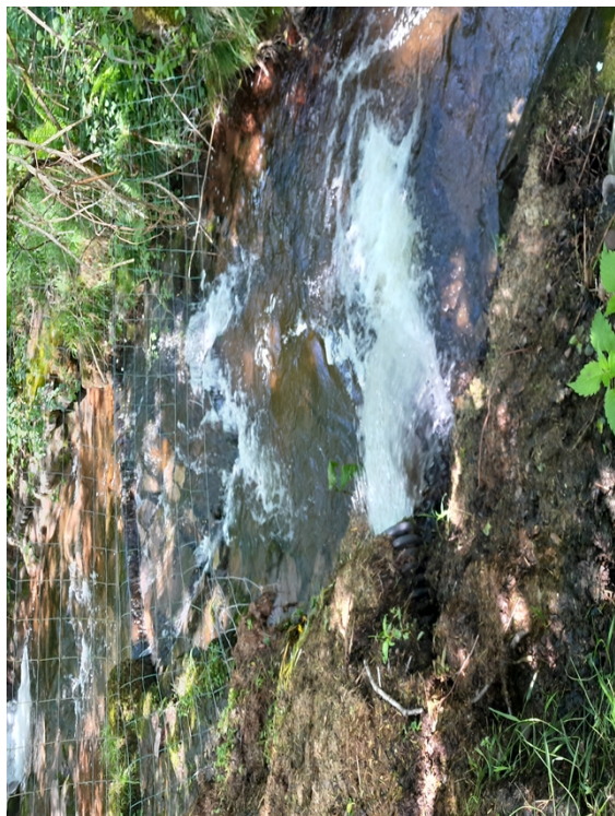
Photograph 1: Shows the discharge point - please install a mesh screen at the end of the pipe.
