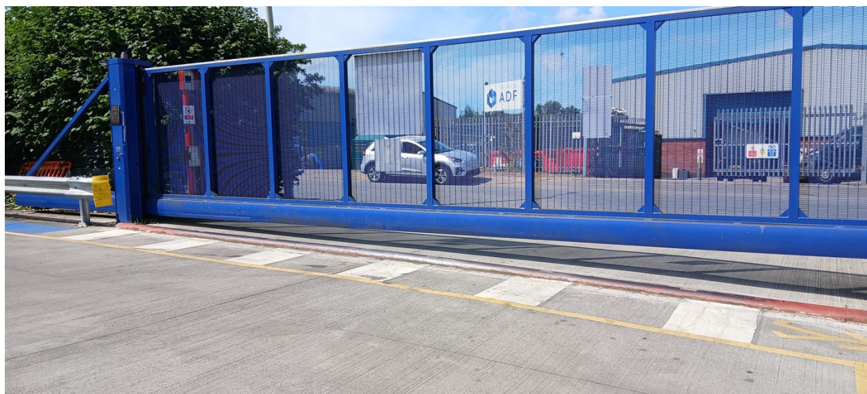
Photo 4 - Raised lip at entrance to site
