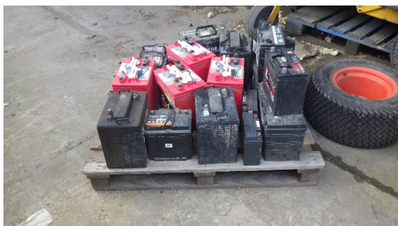
Batteries stored on a pallet
