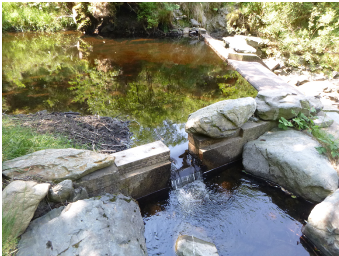
Photograph 1: Hands off Flow notch 6th July 2018.
