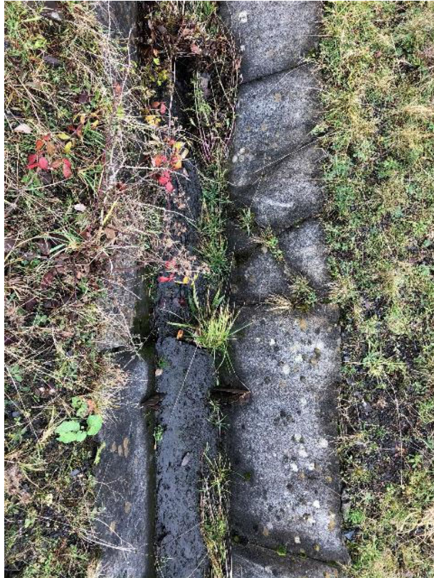
Cracks in concrete drainage channel
