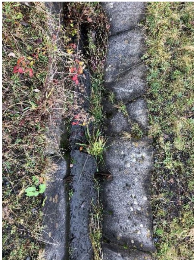
Cracks in concrete drainage channel
