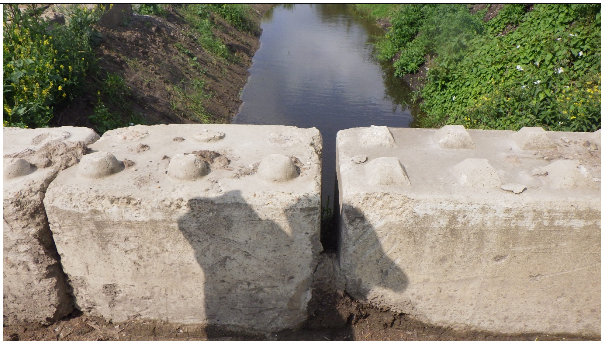
Gaps in blocks
