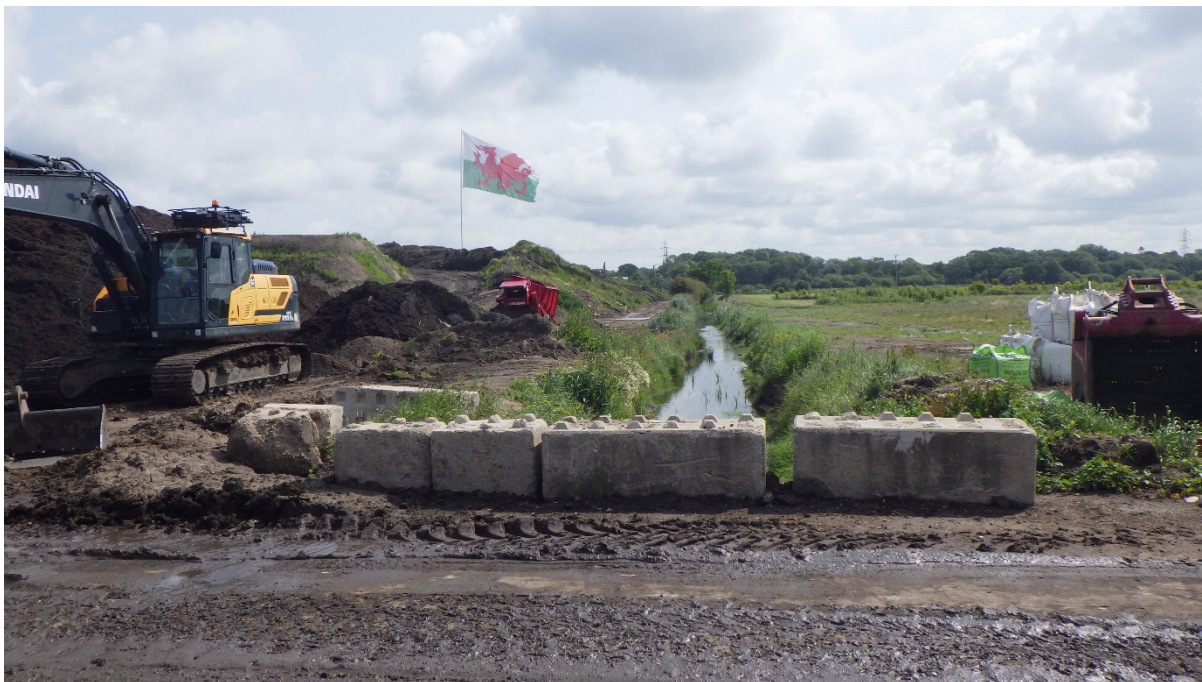
Bridge over Yew Tree brook, not sealed.
