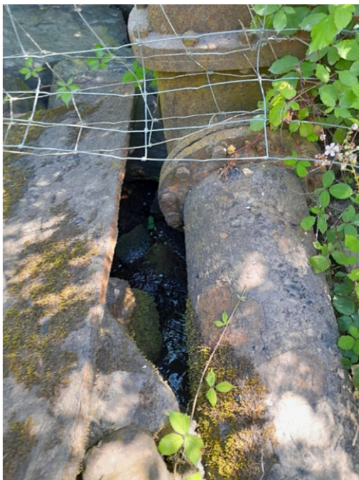
Photograph 4: Flow Under Discharge Pipe
