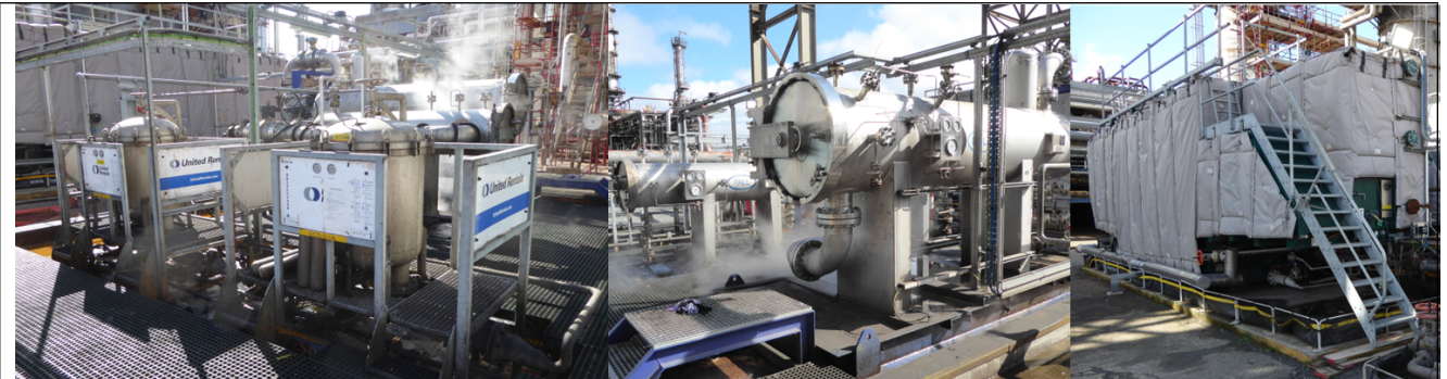
Coalescer, filters and temporary tanks
