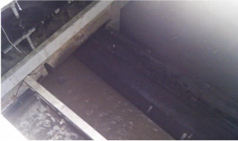
Figure 5: Internal View of Screen Chamber
