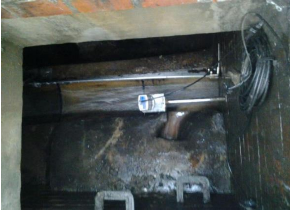
Figure 5: Internal View of CSO chamber and CELLO
