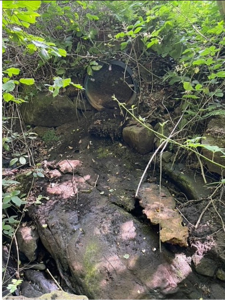
Figure 3: Pumphouse-Discharge outlet with screening
