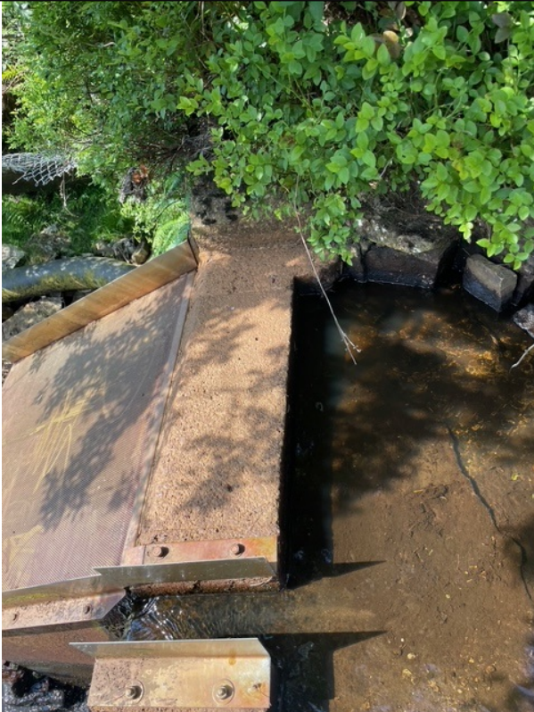
Figure 3: Intake Works- HOF Notch & Perforated Intake Screen
