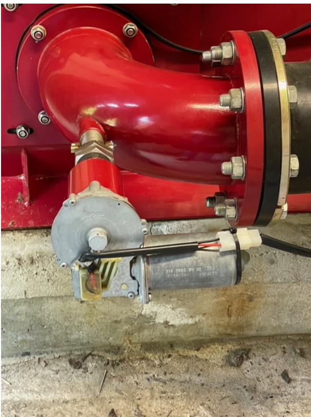
Figure 4: Intake Works- Spear Valve in Pumphouse
