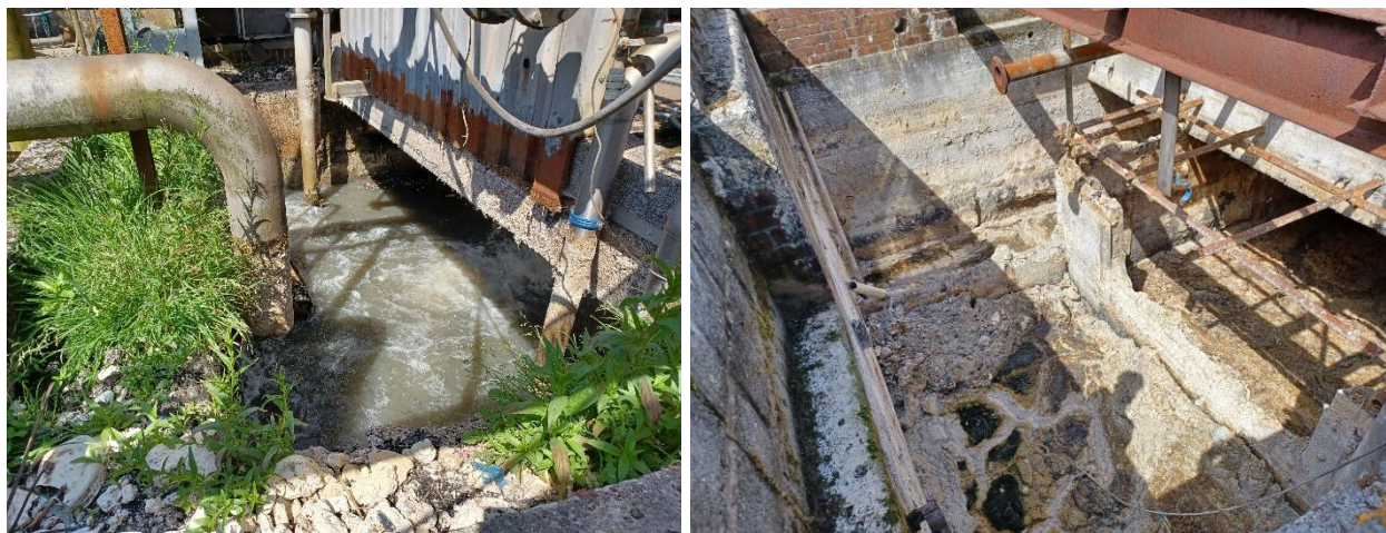
Image 9 & 10: From surface view of Reception Pit (left) and Detritus Pit (right)
