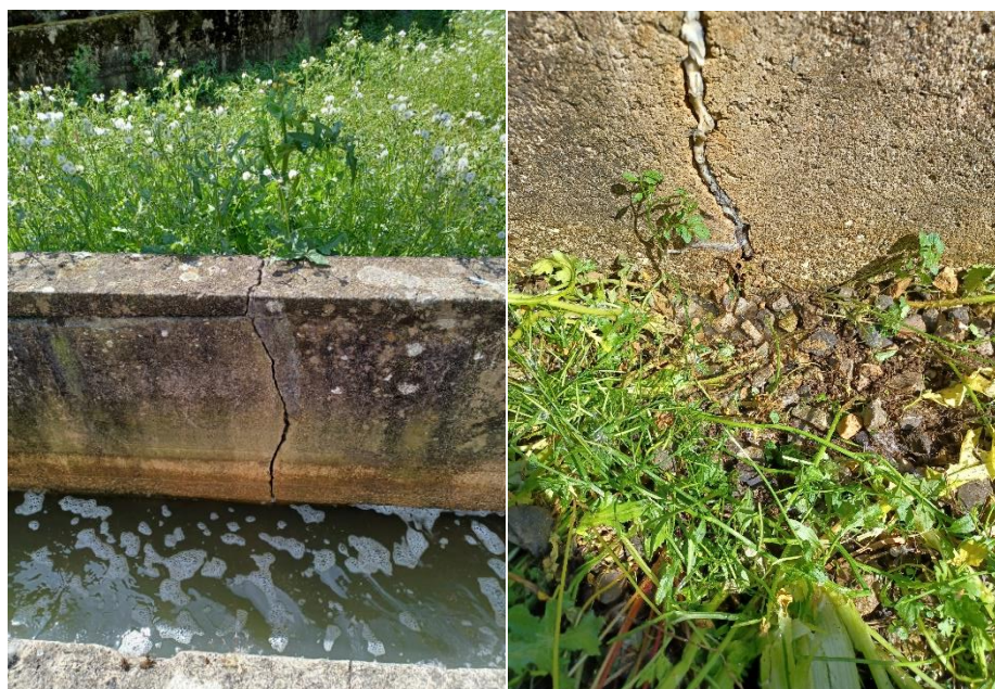
Images 7 & 8: Structural failure of transfer flume associated with the ETP (left) and evidence of loss of containment (right)
