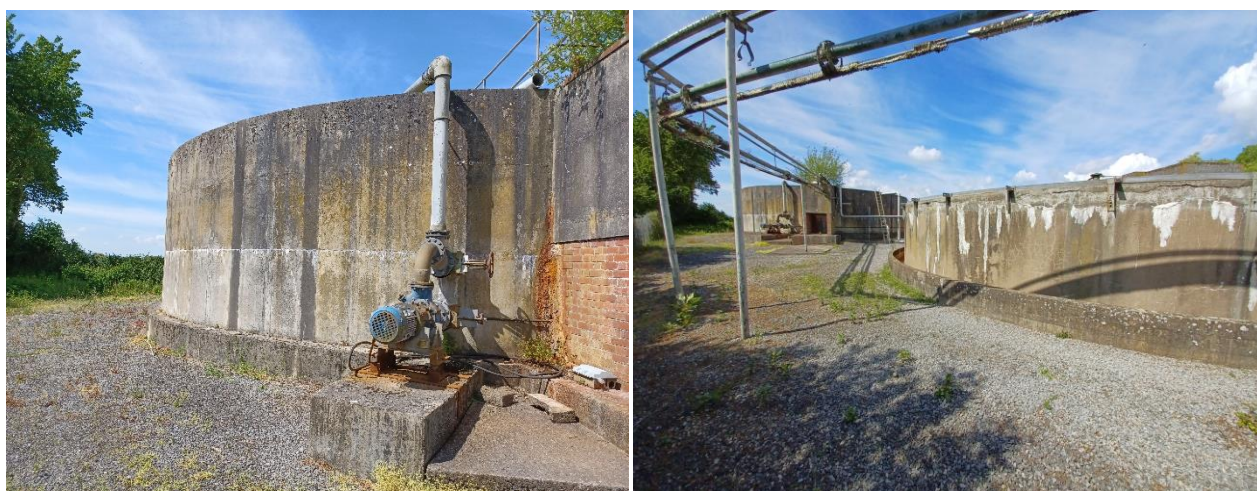
Images 3 & 4: Permeable ground surrounding LUBEK Tank (left) and Rotary Filter Bed (right)
