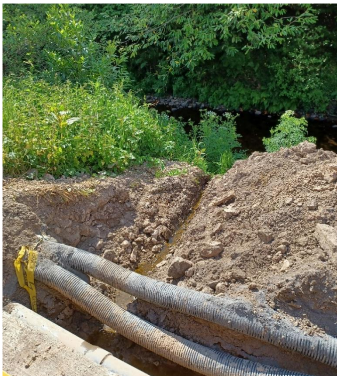
Image 5: Loss of containment from failed Retort Water Pipework into the Afon Bran
