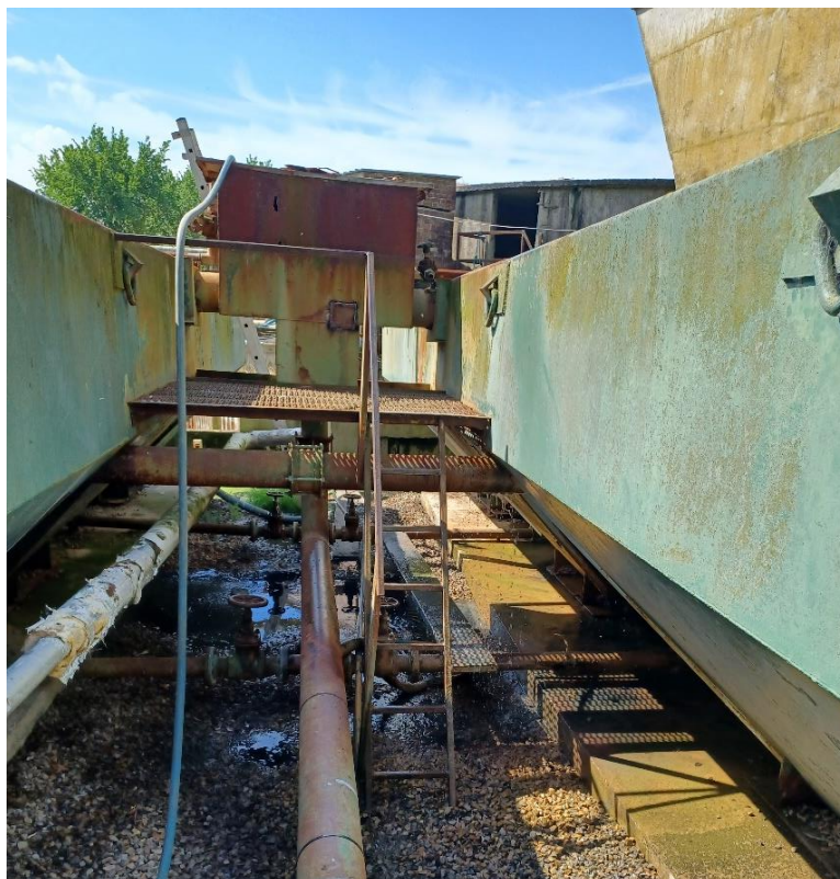
Image 6: Discharge of partially treated effluent to ground from pipework associated with Final Clarifiers
