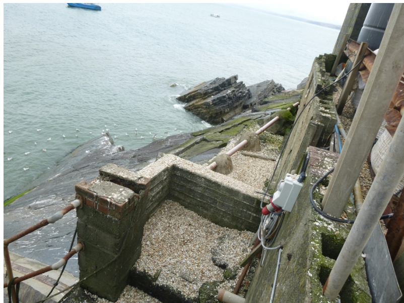
Photograph 1: Final effluent discharge pipe into New Quay Bay
