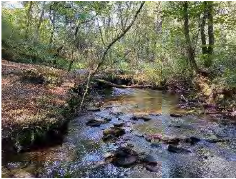
Photo looking up stream Nat y Gaeltach. River runs through 3no. Ducts whilst passing under farm track. River diameter approx. 6 m. Moderate Flow
