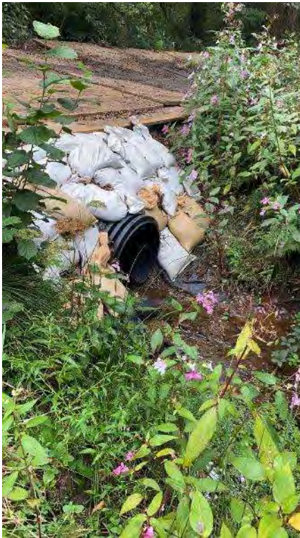
Stream running under temporary road surface. Low velocity and draining towards main river.
