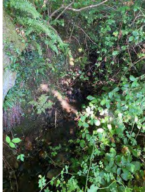
Small stream (width – 0.2 m) with very little water running underneath B road near to Gadlys Farm.
