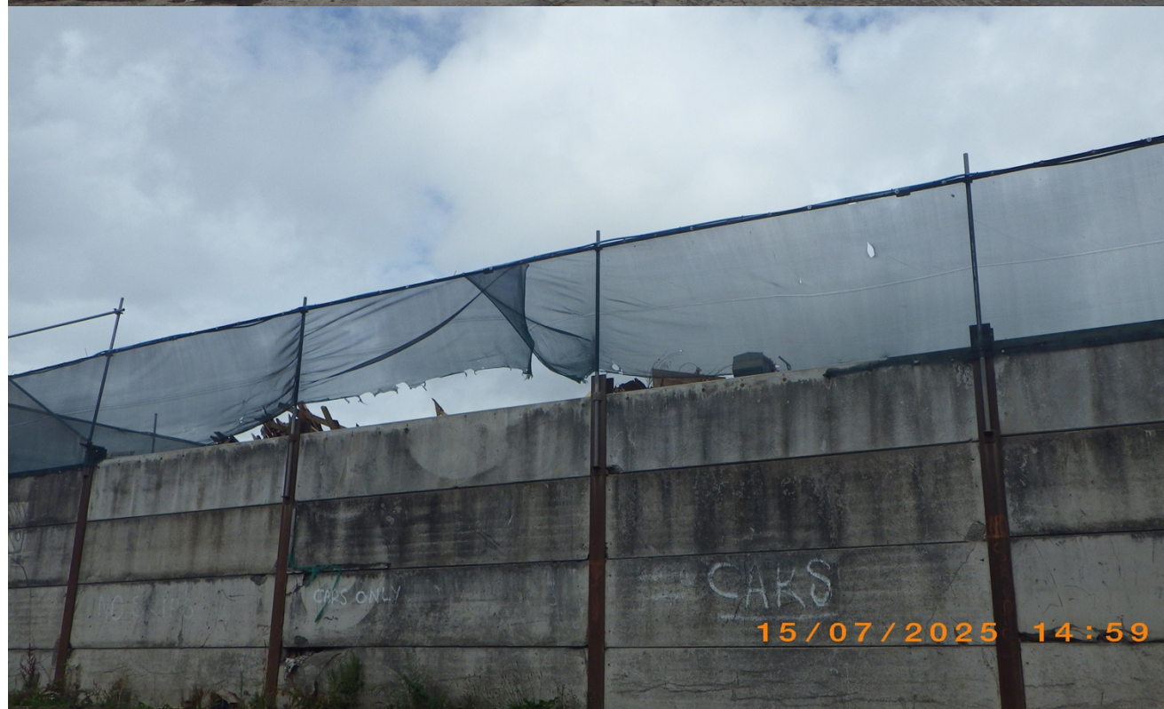
Netting on site boundary showing damage/disrepair.
