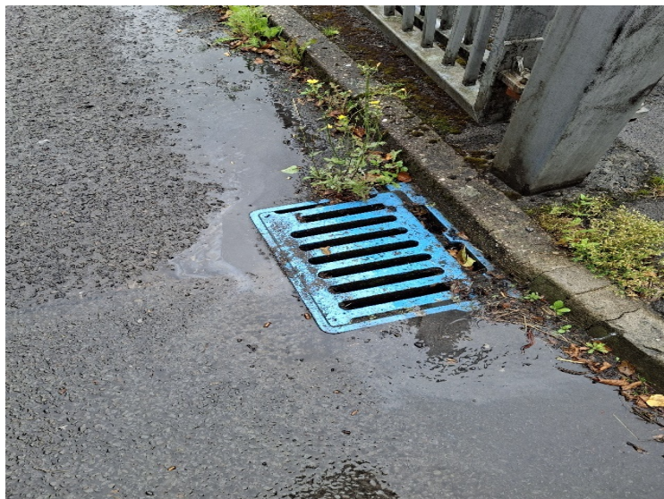
Figure 3: Surface water drain with oil around it
