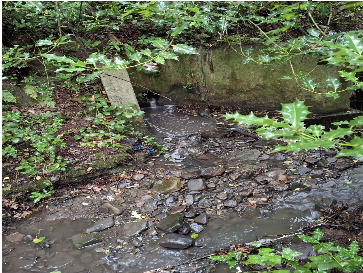
Figure 1: Discharge point into the tributary
