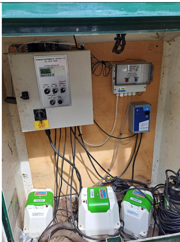
Figure 6 – The treatment plant control box as observed during the visit.
