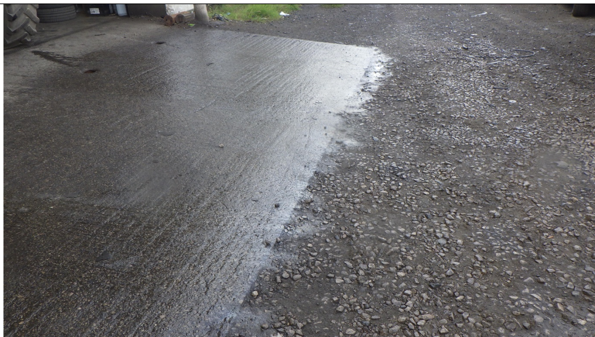
Older de-polluting building oily run off.
