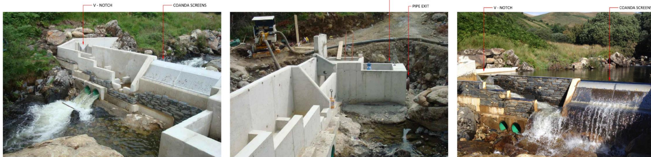
WEIR: Micro Hydro, 375kW Cadair Hydro (150m head, 300l/s, pelton turbine), operated by Dragon Hydro www.dragonhydro.com Photos: Jonathan Bensted
