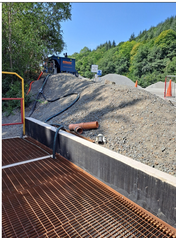
Figure 9 – The treatment system used to treat drainage effluent from the final catchment weir.
