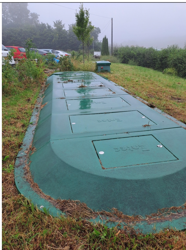
Figure 7 – The old treatment system as observed during the visit.
