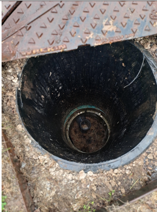
Figure 1 – Primary solids separation chamber as observed during the visit.
