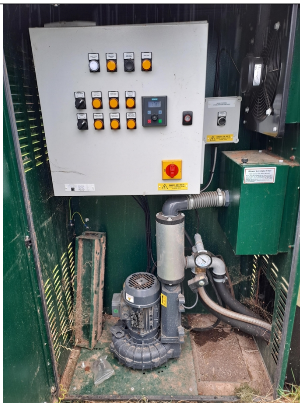
Figure 4 – The treatment system control box as observed during the visit.
