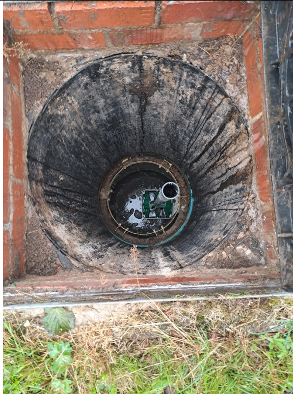
Figure 3 – Final treated effluent chamber as observed during the visit.
