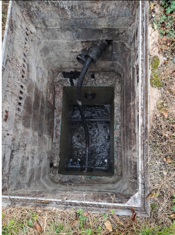
Figure 2 - Aeration and bio media chamber as observed during the visit.
