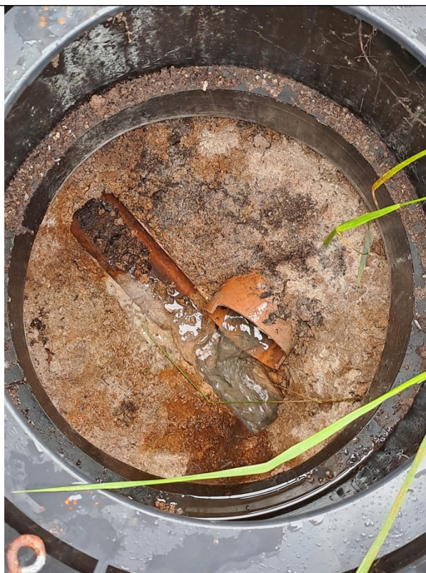
Figure 6 – The observed sample point at the time of the visit. Consistent clear flow can be see discharging. Note the defunct and isolated input from the old system in the top left of the chamber.
