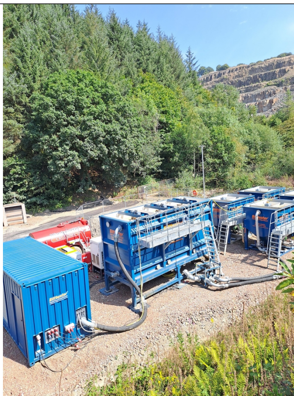
Figure 6 – An overview of the water treatment system infrastructure.
