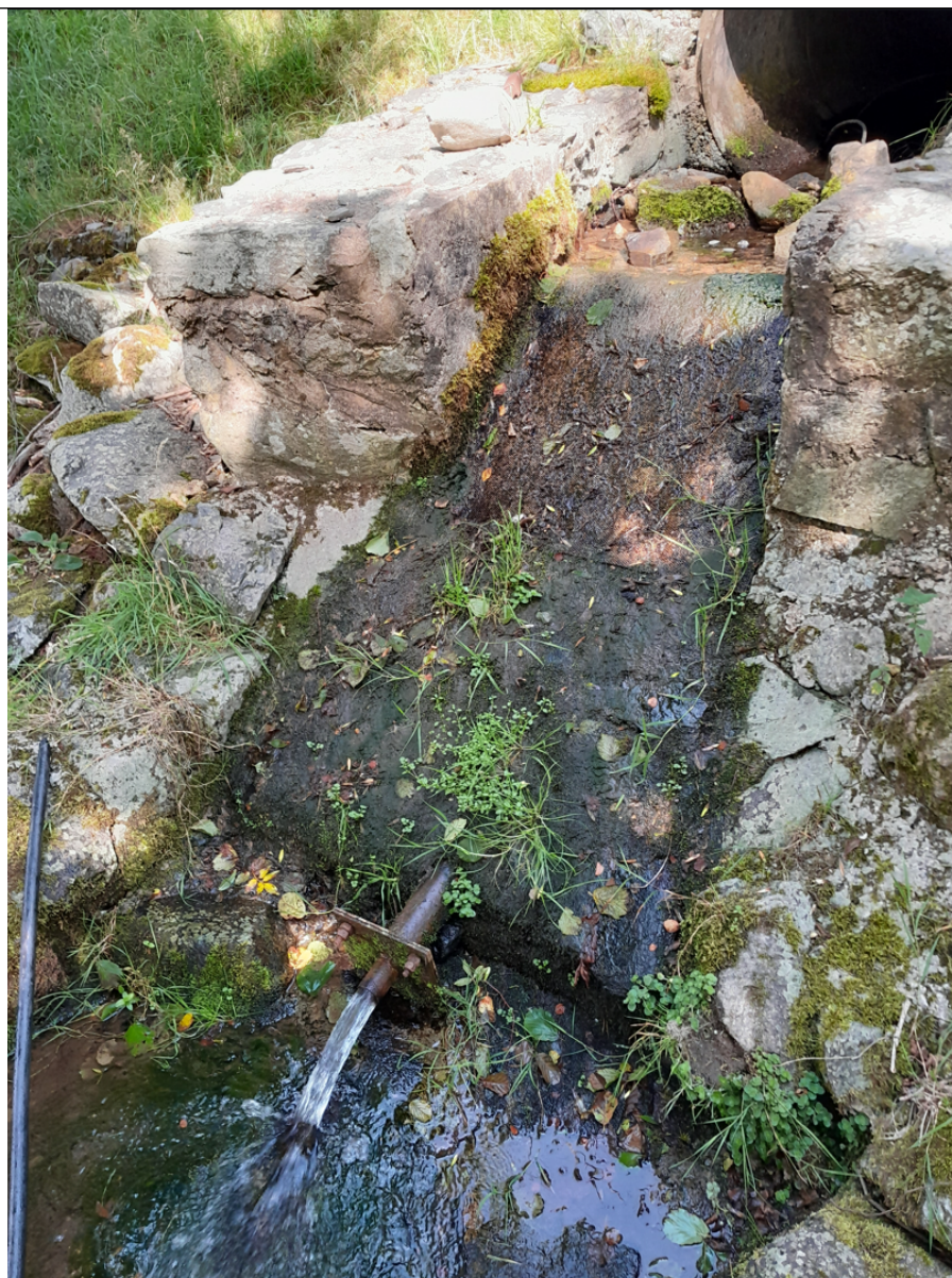
Photo 1 Intake screen and by-pass flow mechanism
