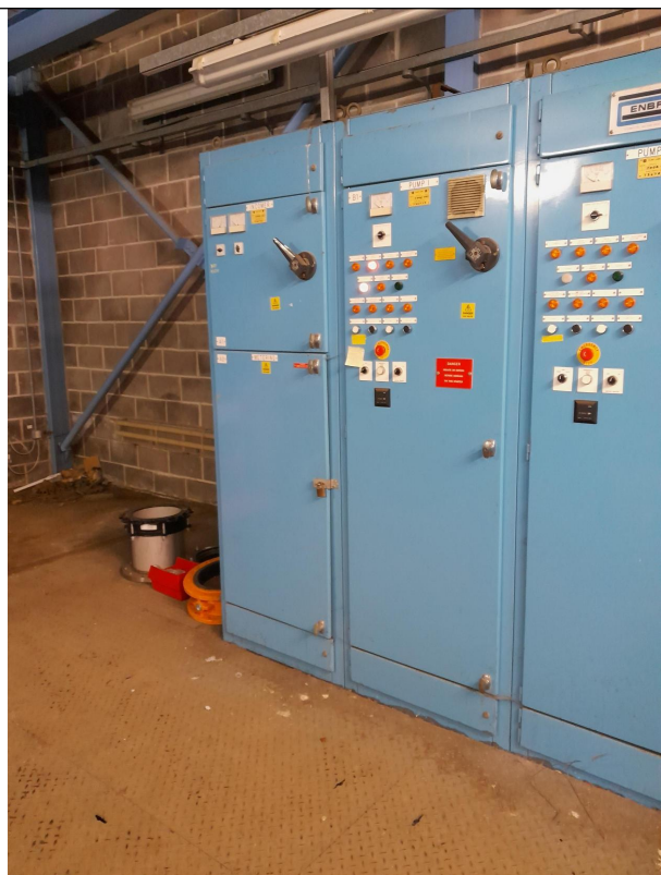
Figure 4: Interior of Dwr Cymru pumping station showing locked meter cabinet
