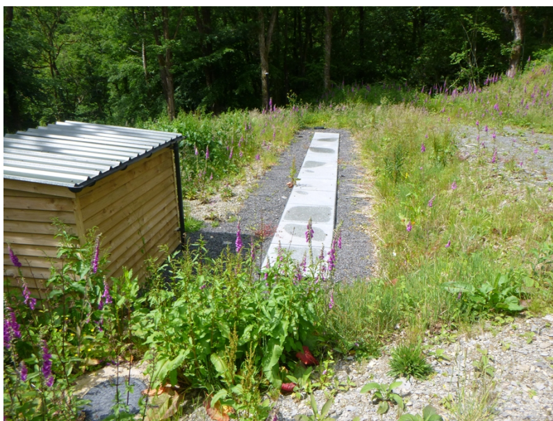
Photograph 1: Package Treatment Plant (PTP) near SN 74329 76974
