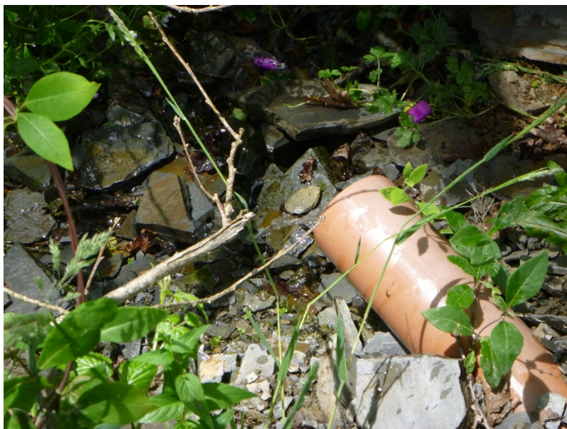
Photograph 3: Package Treatment Plant (PTP) outfall
