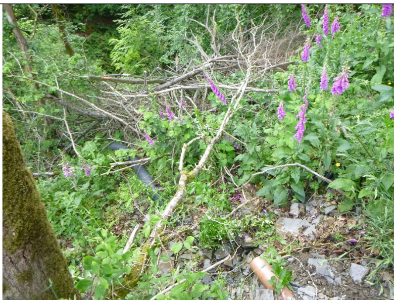
Photograph 4: Package Treatment Plant (PTP) outfall
