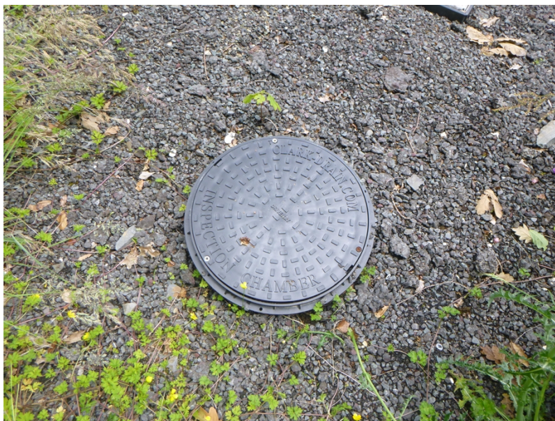
Photograph 2: Final effluent inspection chamber
