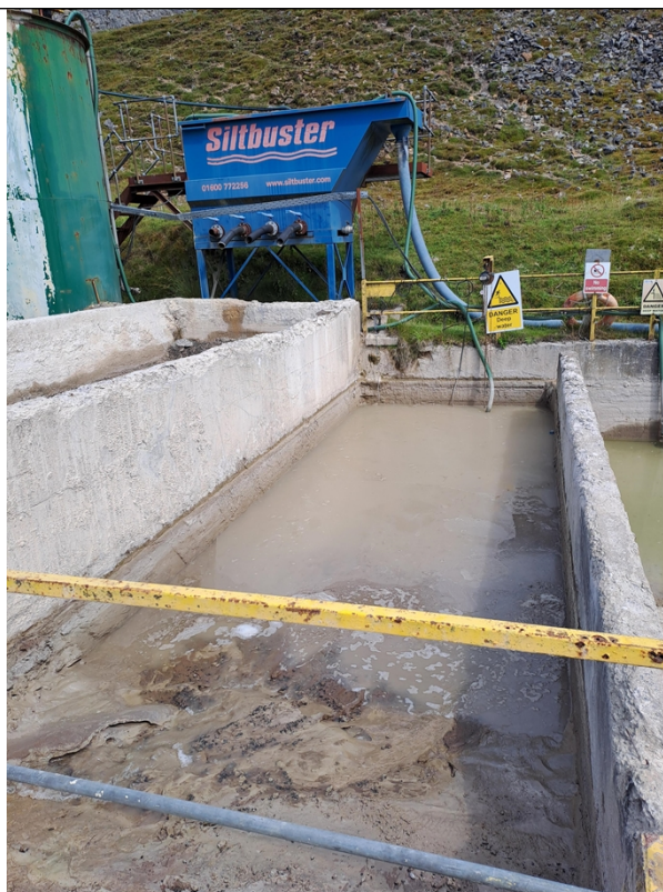
Figure 4 – The dirty/primary settlement pit as observed during the visit.
