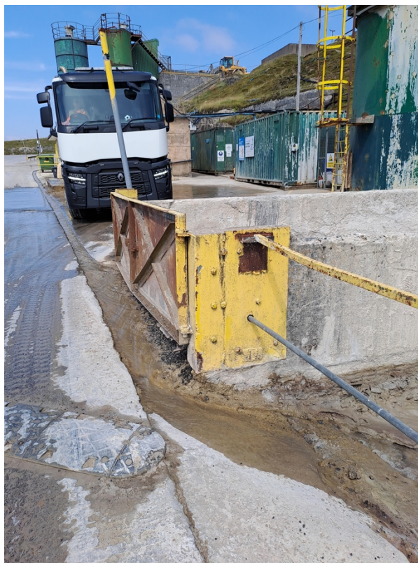
Figure 3 – Wash out water from a mixing vehicle entering the settlement pit via drainage channel as observed during the visit.
