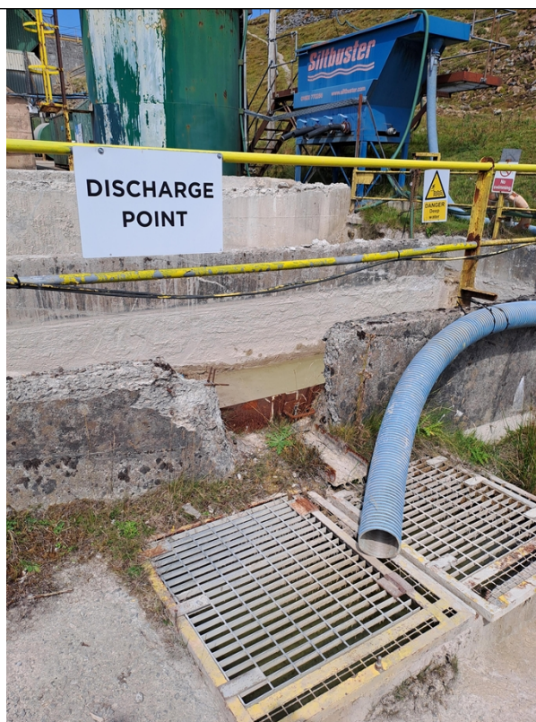
Figure 6 – The discharge/sample point as observed during the visit.
