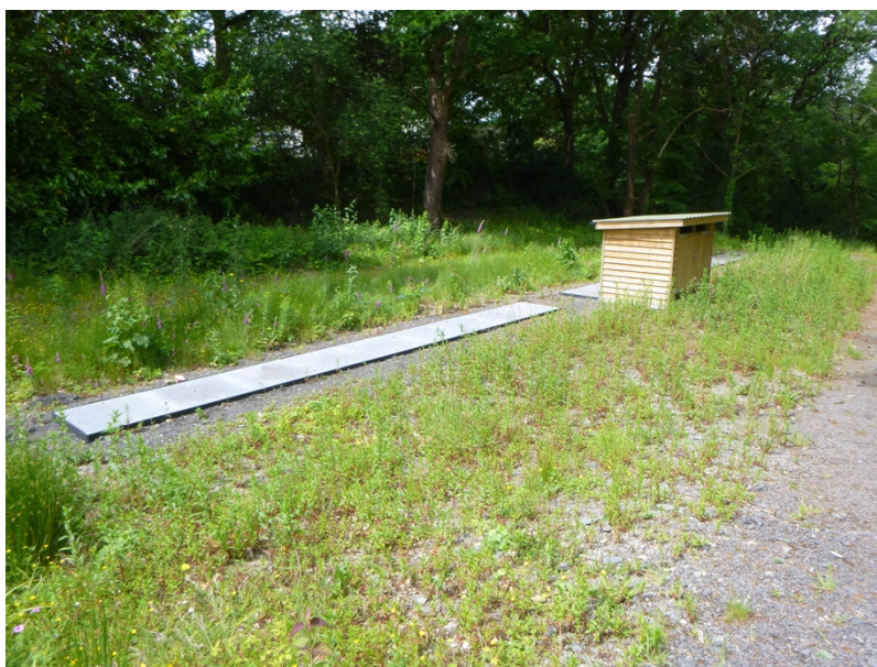
Photograph 1: Package Treatment Plant (PTP) near SN 74560 77385
