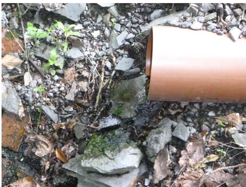
Photograph 3: Package Treatment Plant (PTP) outfall
