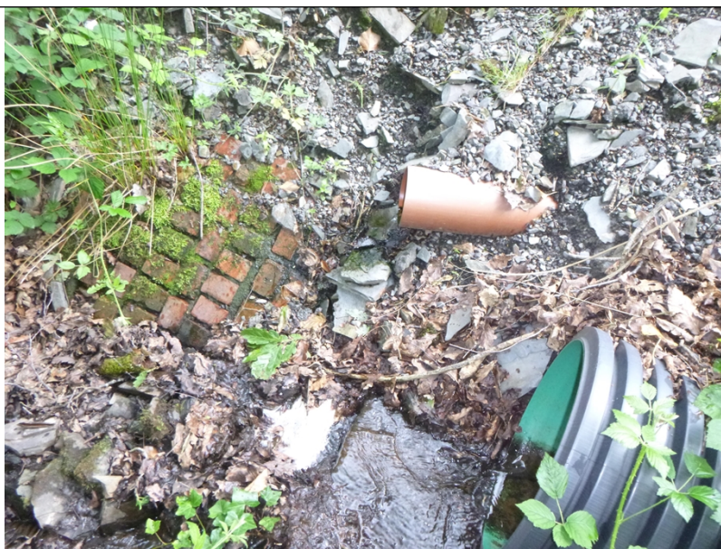
Photograph 4: Discharge from Package Treatment Plant (PTP) entering unnamed watercourse
