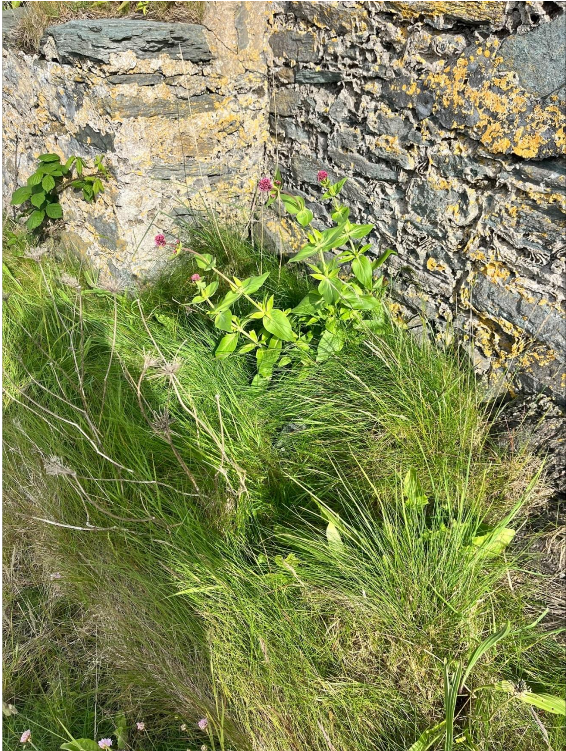
Photograph 3: Vegetation growing from the east side of the bridge at the top of the retaining wall.
