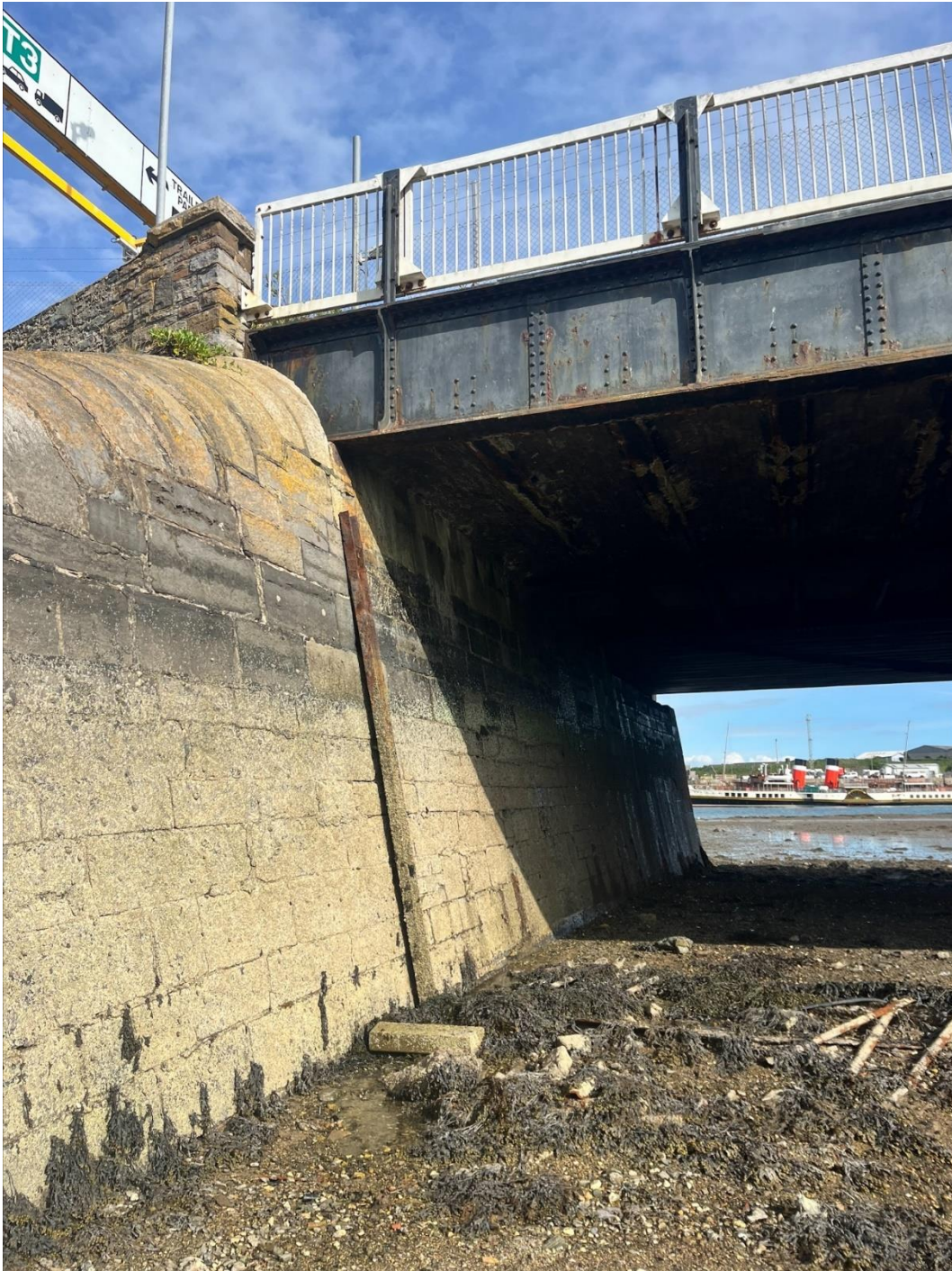
Photograph 5: Viewing from underneath the bridge facing North East and view of debris to be removed.
