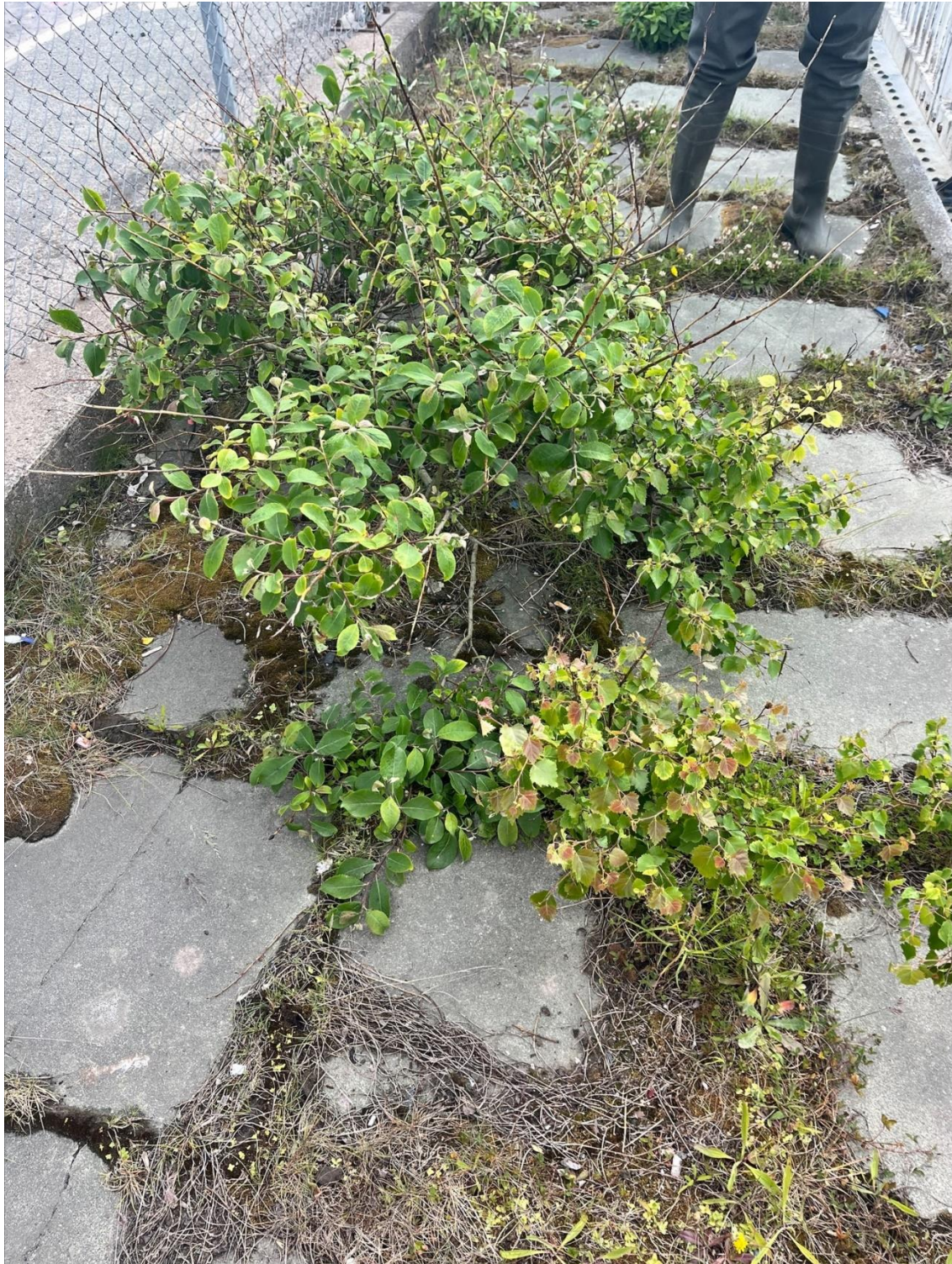
Photograph 2: Vegetation including birch and willow saplings growing from the deck.
