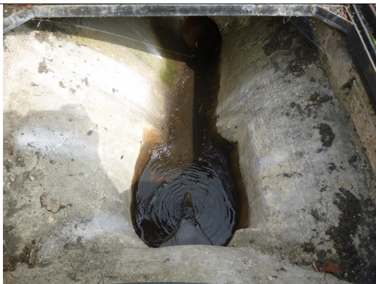
Photo 2: Final effluent sampling point with sewage fungus present in the channel
