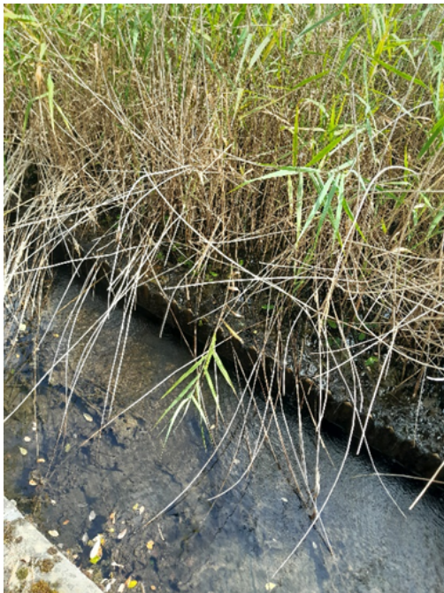
Photograph 3: Sludge Build Up at Reed Bed Outlet
