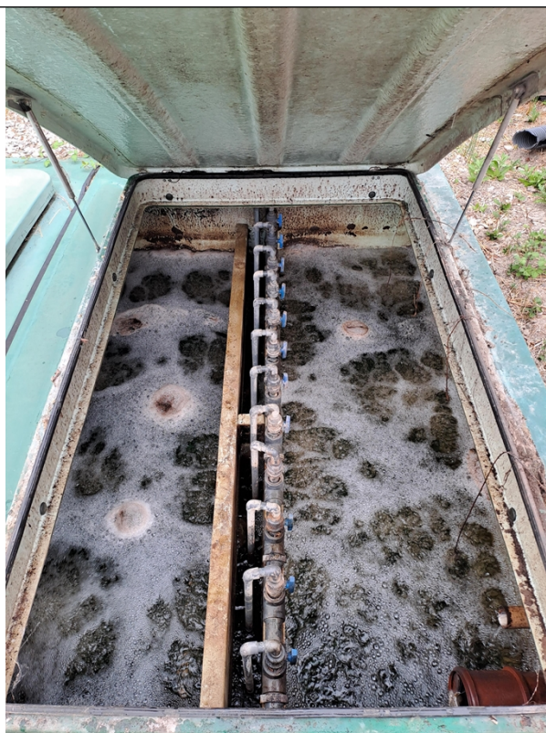
Figure 3 – The aeration chambers as observed during the visit.
