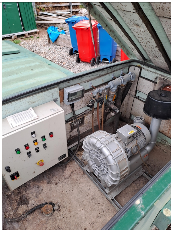
Figure 5 – The pump and control box as observed during the visit.
