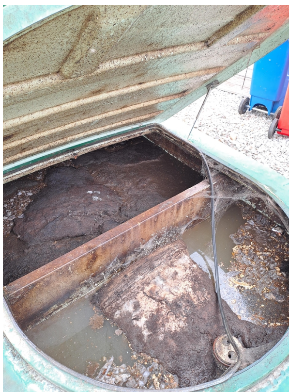
Figure 2 – The primary solids settlement chamber as observed during the visit.
