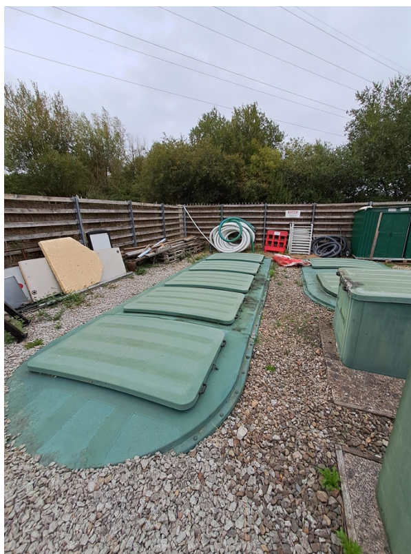
Figure 1 – The sewage treatment infrastructure as observed during the visit.
