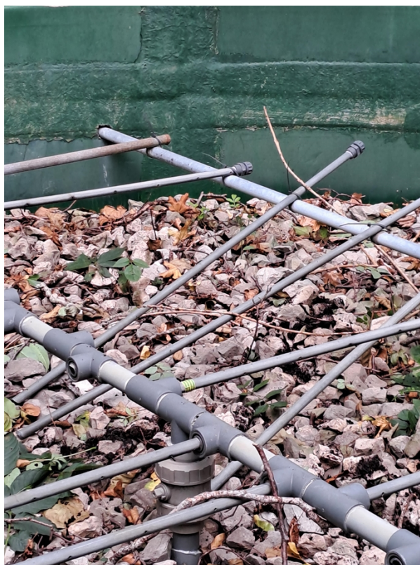
Figure 4 – The filter system as observed during the visit. Damaged spray bars as described above.
