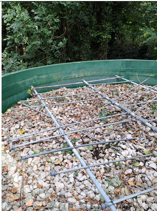
Figure 3 – The filter system as observed during the visit. Damaged spray bars and vegetation build up clearly present.
