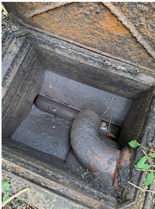
Figure 5 – The final effluent sample point as observed during the visit.
