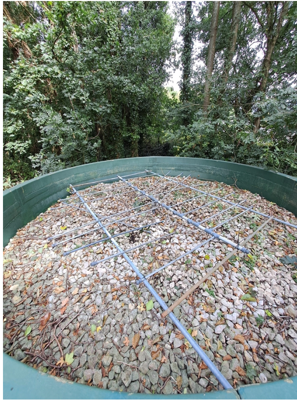
Figure 2 – The filter system as observed during the visit.
