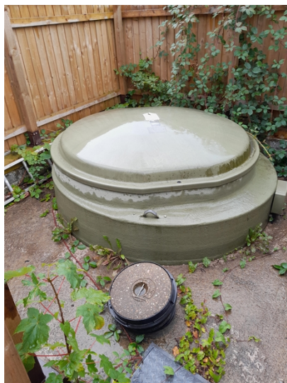
Fig 1 (Kee Sewage Treatment Plant)
