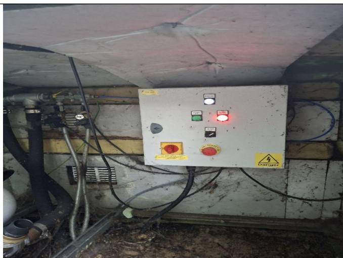
Figure 4: Control panel indicating that the blower had tripped
