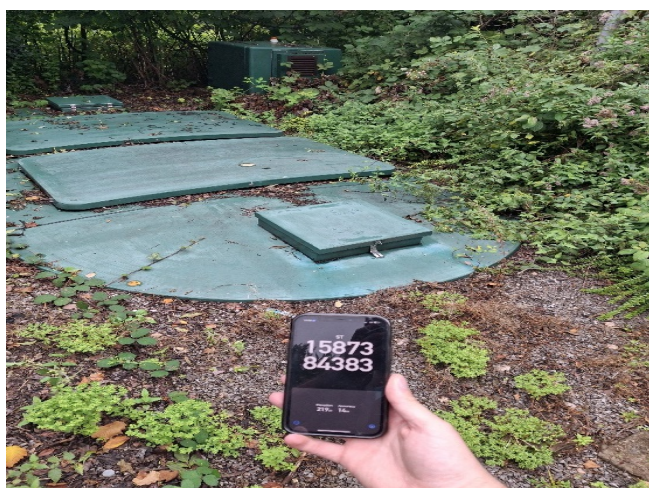
Figure 5: External view of the treatment system
