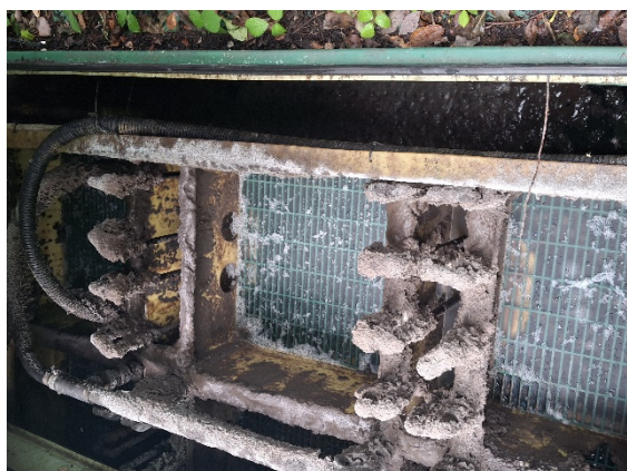
Figure 7: Second chamber of the system with blowers inactive
