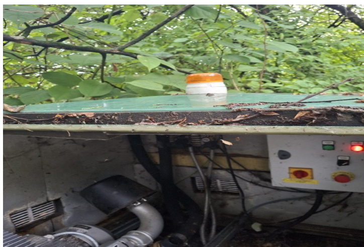
Figure 3: Flashing alarm indicating an issue with the system
