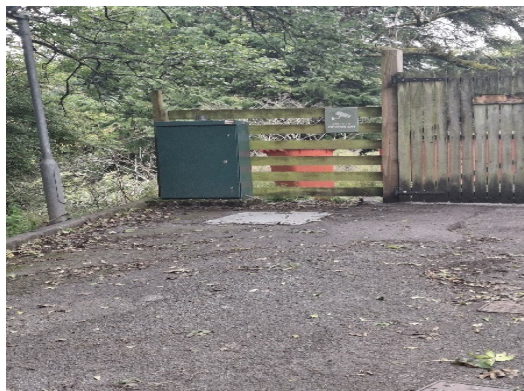
Figure 1: Lower alarm indicating system fault
