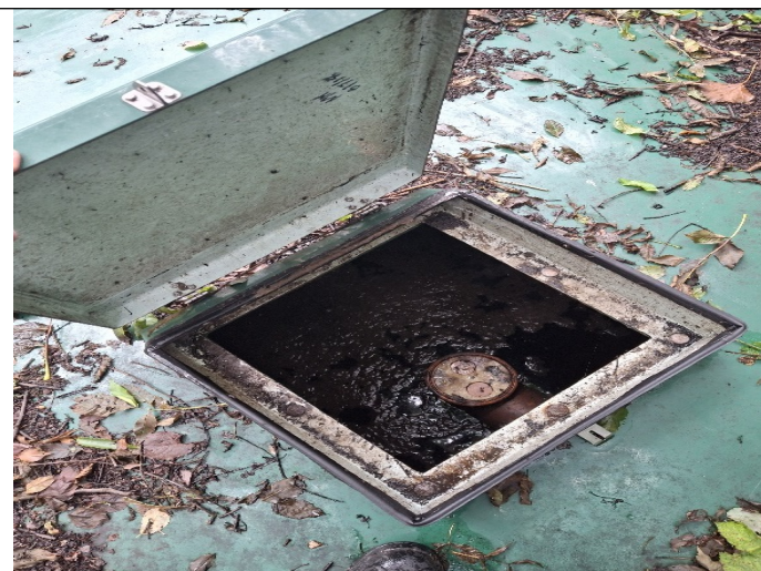
Figure 6: Initial chamber of the system showing high amount of solid waste
