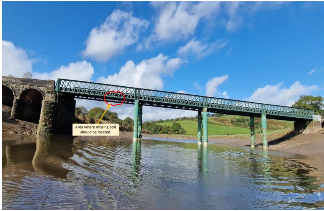
Photo highlighting missing bolt.
