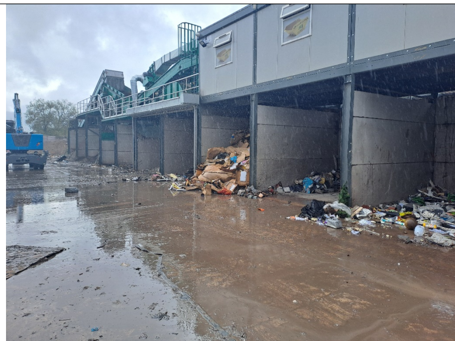
Photo 3 - Bays for sorted material
