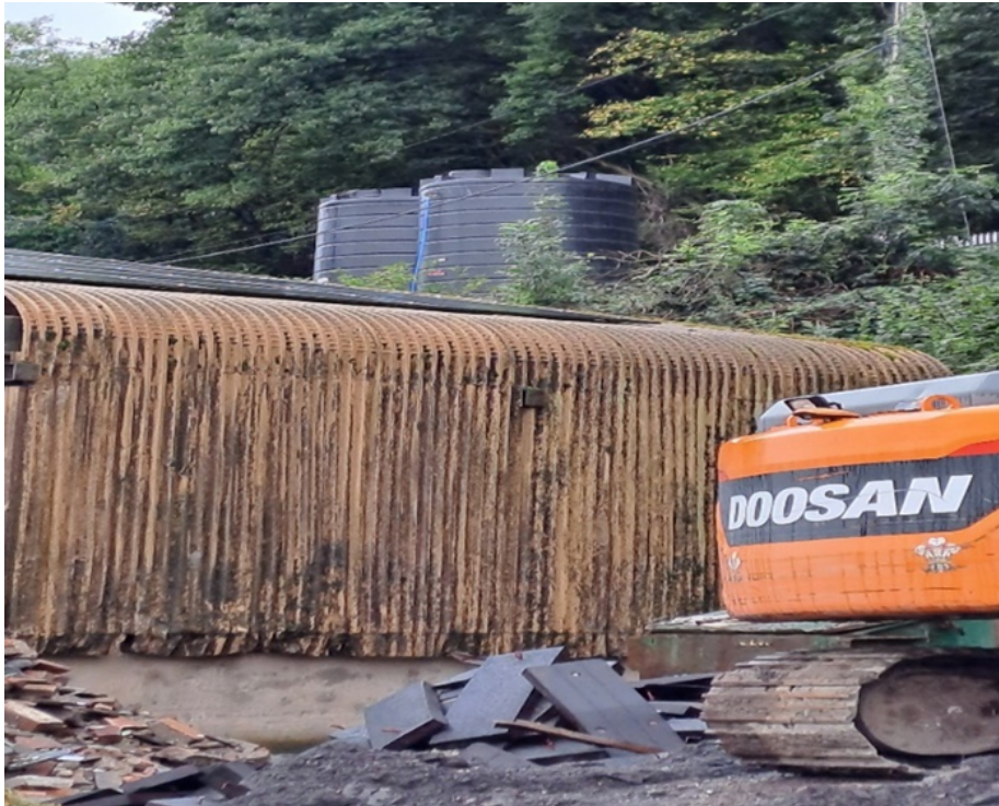
Photo 1 – Water tanks at CWS Ltd with increased capacity for dust / fire mitigation
